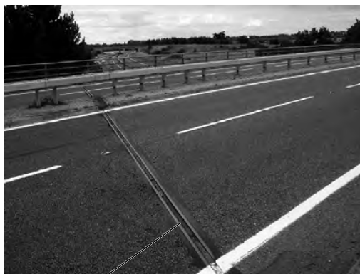
gap in bridge
